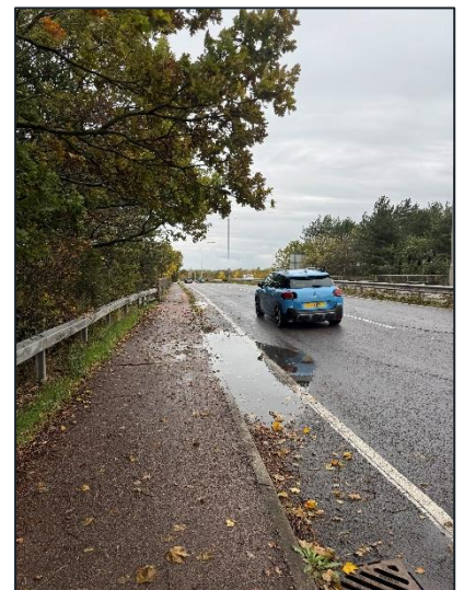
Surface Water Pooling
