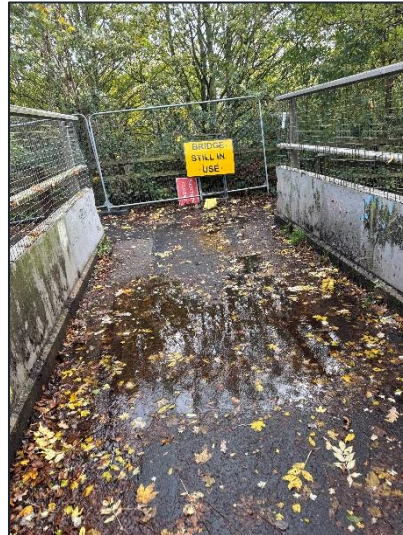
Surface Water Pooling
