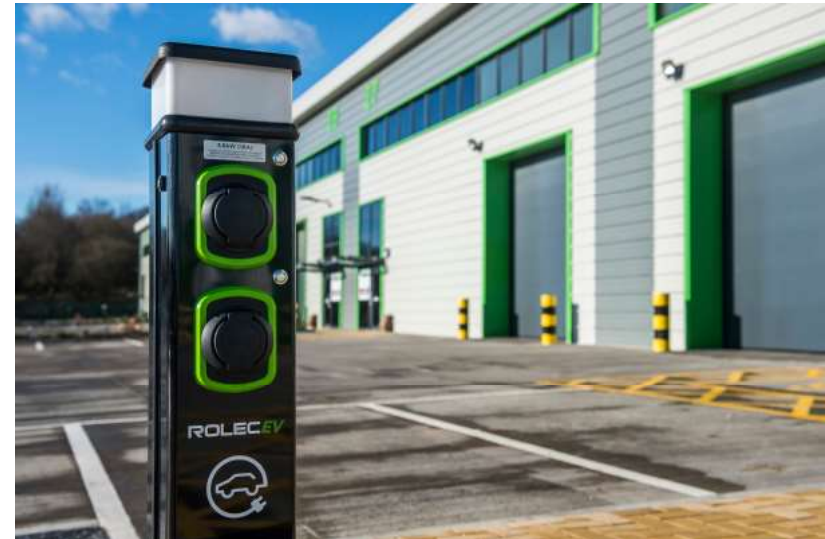
ILLUSTRATIVE VEHICLE CHARGING POINT
