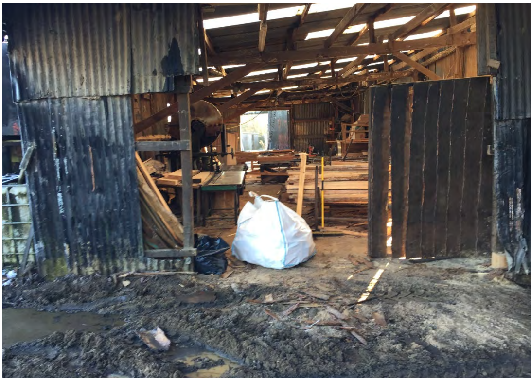
Fig 16 – Internal of machinery building
