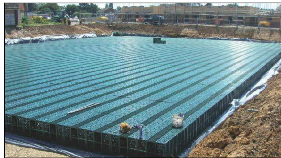
CELLULAR STORAGE TANKS: CELLULAR STORAGE TANKS PROVIDE AN EFFICIENT MEANS OF SURFACE WATER ATTENUATION AND ARE TYPICALLY LOCATED BENEATH LARGER PAVED AREAS. TANKS DO NOT PROVIDE A LEVEL OF TREATMENT.
