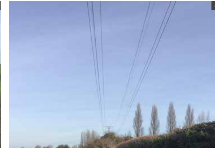
High voltage power cables follow the alignment of hedges and ditches
