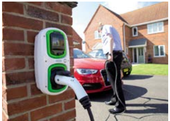
Electric charging infrastructure for new homes.
