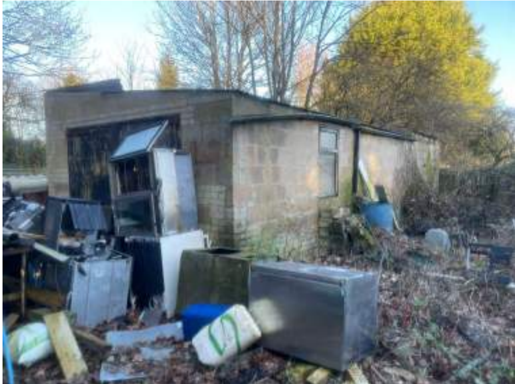
Photograph 6. Ruined building with damaged roof in the far west of the Site.
